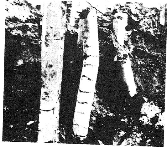
Photo 4. Broken RC Piles (H Bldg.)
