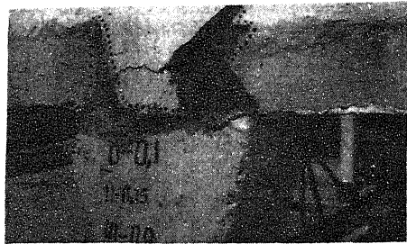
Fig. 4 - Detail of joint cracking.
