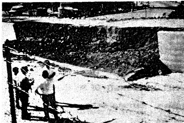
FIGURE 3. PHOTOGRAPH OF TOPPLED OPEN CHANNEL WALL.
