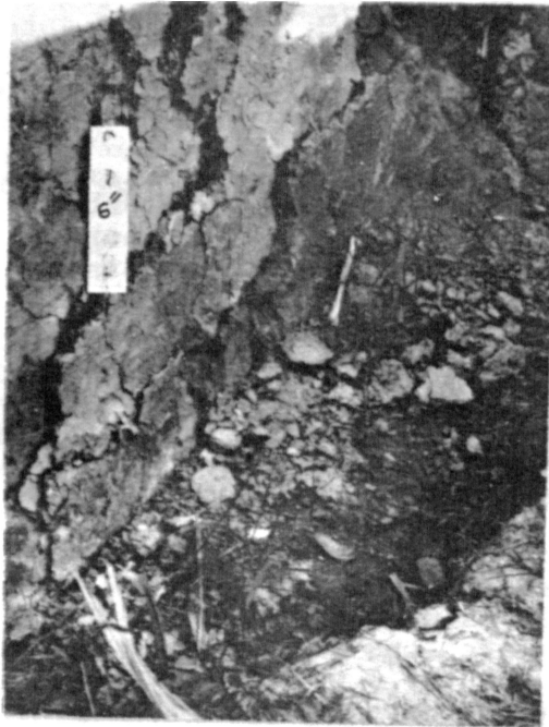
FIG. 5 - WIDE CRACKS AND PARTIAL COLLAPSE OF MUD WALL NEAR POHANA VILLAGE
