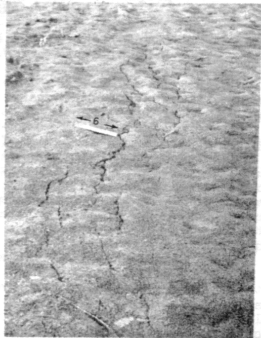
FIG. 6 - DEVELOPMENT OF FISSURES ON THE BANK OF SOLANI RIVER ABOUT 8 km S.E. OF ROORKEE
