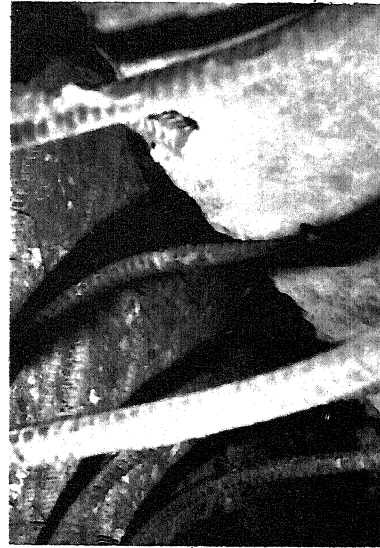
Photograph Number 2. Close-up of west wall failure at base of wall. Rebar is inner face wall reinforcing. Horizontal break in concrete occurs at top of dowels.
