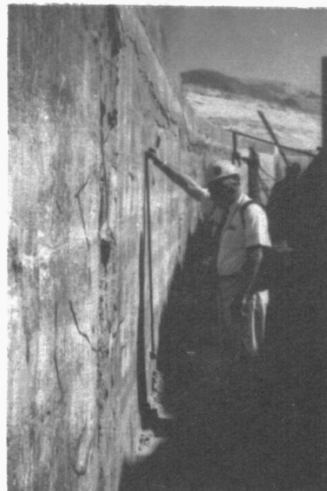
Photograph Number 10. East of wall of Effluent Conduit in "S" curve area after backfill removed. Note out of plumb of wall, which was 4 inches maximum for 8-1/2 foot inside height.
