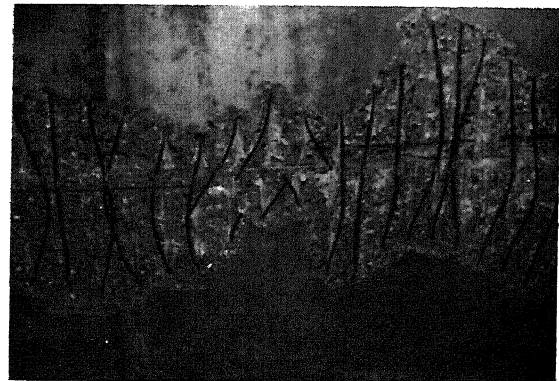
Photograph Number 4. Construction joint on line 24-1/2 where three reinforcing bars failed by necking in tension. Measurements indicated that the joint slid a minimum of 15 inches one way, 11 inches the other way.
