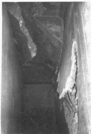
Photograph Number 7. East wall of reservoir near line 24 looking north. Wall at left is cantilever overflow wier wall. Note slab failure above.
