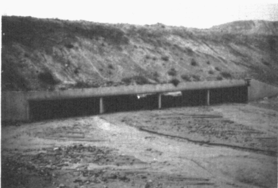
Photograph Number 11. Box Culvert for railroad spur line looking north. Culvert is half full of mud and silt. Culvert racked to east or right by 4 to 6 inches.
