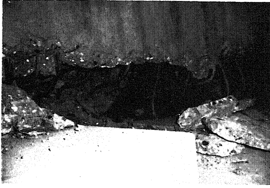
Photograph Number 1. West wall of reservoir failed at its base. Wall has pushed in and dropped. Concrete in foreground is floor slab drop panel.
