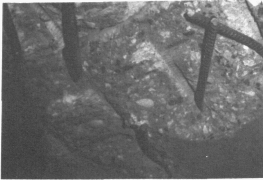
Photograph Number 5. Close-up of broken reinforcing bars in Photo Number 4. Note tension failures of reinforcing and scratch marks of deformations on bars on the concrete surface.
