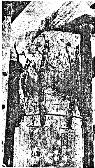
Fig. 9 - Column Failure, Marco Aurelio Building
