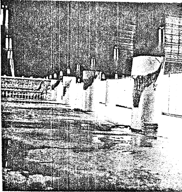
Fig. 5. Macuto Sheraton's mezzanina damaged columns.
