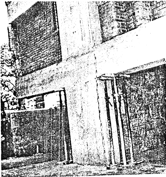
Fig. 7. Petunia I, South front. Beam with shear damage.
