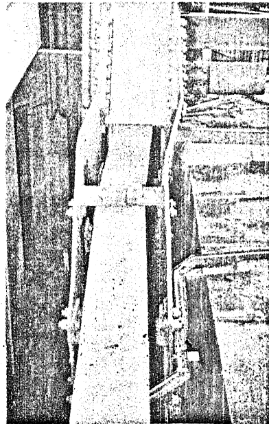
Photograph No 4 Boiler Structure diagonal connection at ----- elevation 75'-5". The girder's lateral deformation and bent gusset can be seen.
