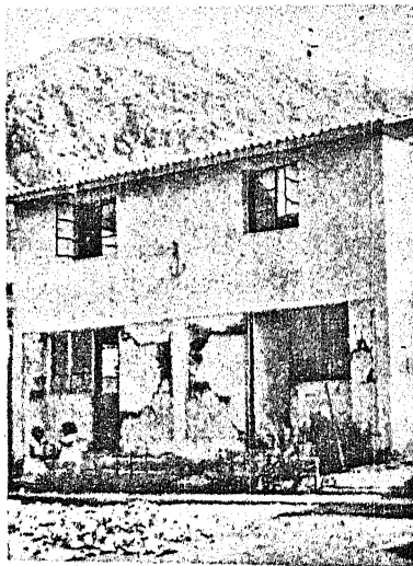
Fig. 5.- Tocopilla, Dec. 20, 1967 Earthquake, MM VII-VIII. Two -story reinforced block masonry house.
