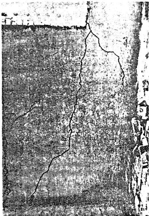
Fig. 4. Damages in the wall of the brick building after the explosion.
