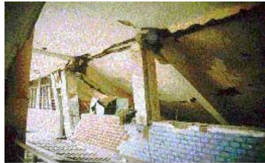
Photo 7: Column failure due to lack of stirrups and confinement
