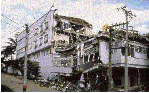
Photo 18: Emergency response teams working in collapsed buildings
