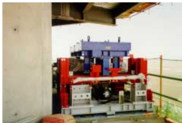
Figure 7. Hybrid Mass Damper installed in the ATC Tower
