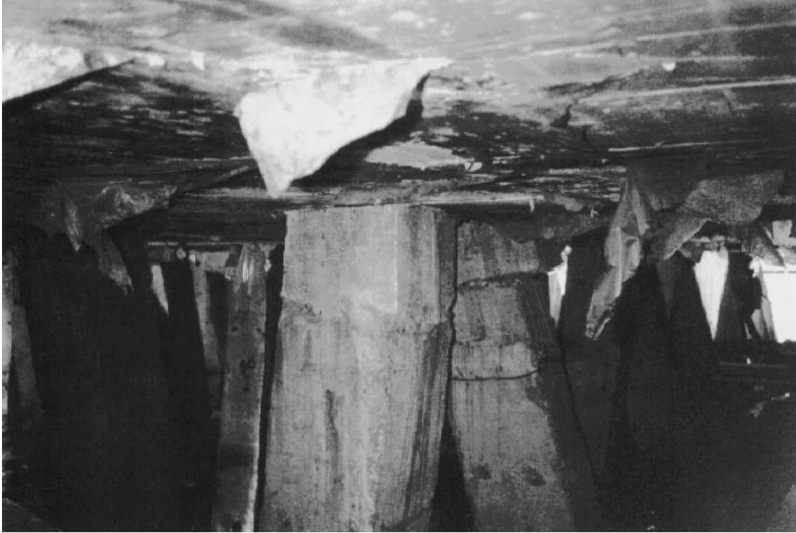
Fig 6. Earthquake induced damage to batter-piles in San Pedrito wharf
