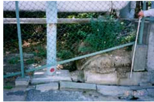
Figure 4: Settlement of the fence near the site
