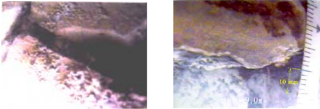
(a) Pile No. 75, depth about 8 m (b) Pile No. 199, depth about 8.5-9.0m Figure 9: Pile damage observed by a CCD camera from inside
