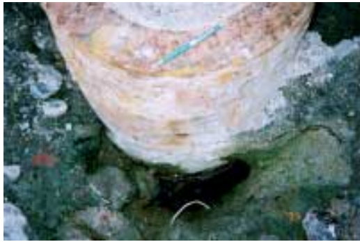
Figure 3: Hole found near pile surface
