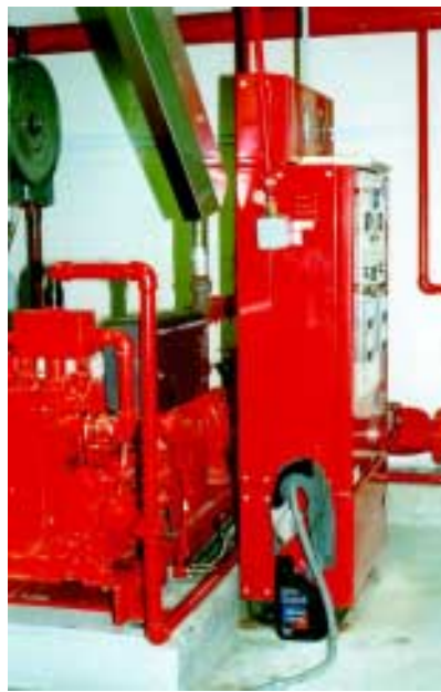
Figure 2 Unrestrained control cabinet for diesel powered emergency sprinkler pump
