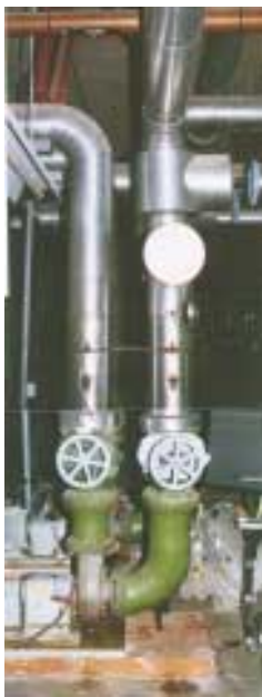
Figure 1 Insufficiently braced pipe work above pumps
