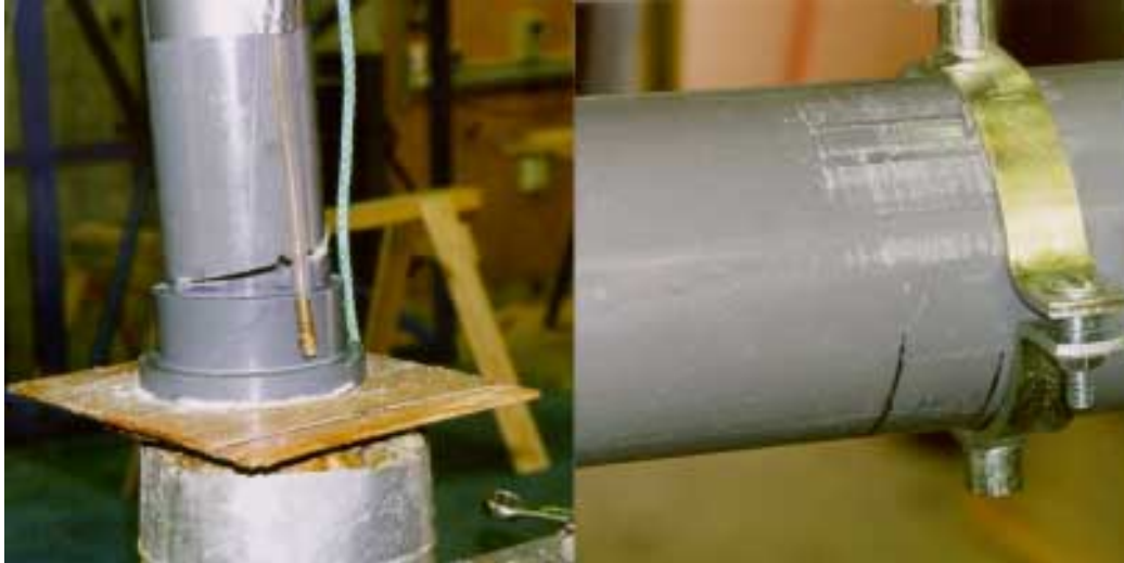
Figure 6 Fractured pipe at flange (flange disconnected) and evidence of support bracket movement on pipe
