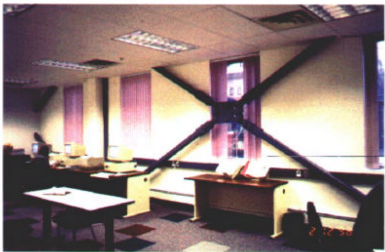
Figure 2 : Harry Stevens Building: Upper Floors X-Braced Dampers
