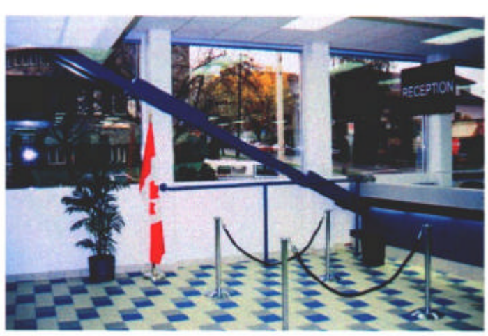
Figure 1 : Harry Stevens Building: Main Lobby with Damper in Lower End of Diagonal Brace
