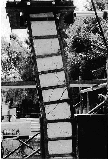
Figure 5: Pattern of cracks
