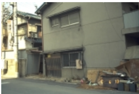
Photograph 1: Inclination damage (inclination angle: 2.0 degree)
