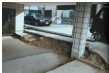
Photograph 2: Subsidence Damage (amount of subsidence: 500 mm)
