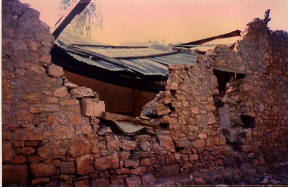
Partial destruction of random rubble masonry wall Fig.1
