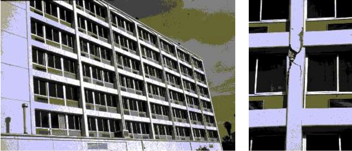
Figure 2: South face of structure (left), and detail of damaged column (right) - damage after the 1994 Northridge earthquake [EERC 1994]
