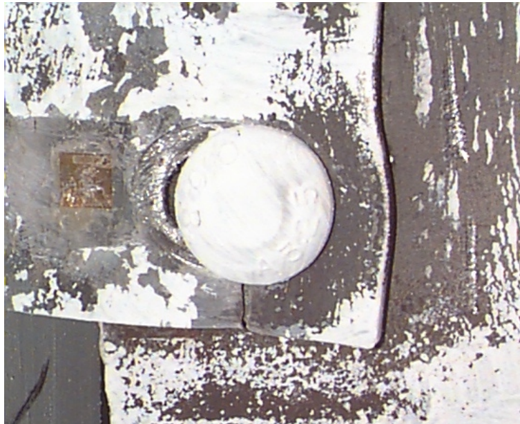
Figure 4: Deformation of bolt hole and fracture, Specimen 2A
