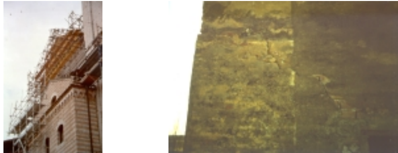
Figure 1: the Bell-Tower of the S. Giorgio in Trignano Church in S. Martino in Rio, damaged during the October 1996 earthquake (right), and the transept tympanum of the Basilica of S. Francesco in Assisi, damaged during the September 1997 earthquake (left).
