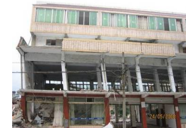
Plastic hinges in frame columns, Nanba
