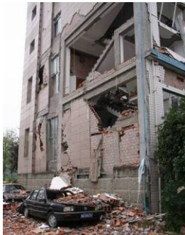
Filler wall collapsed, Dujiangyan
