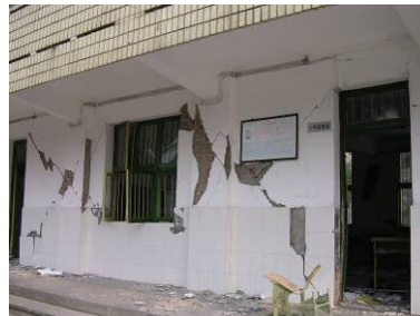
Severe damage in the load-bearing walls and columns of the teaching building of Huayuan St. Middle School, Jiangyou
