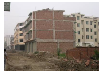
Undamaged masonry structures with concrete structural columns and ring beams in Anxian
