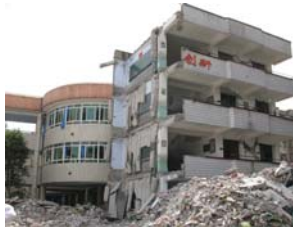
Figure 8. Collapsed primary school
