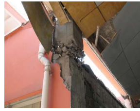
Figure 10. Column flexural failure
