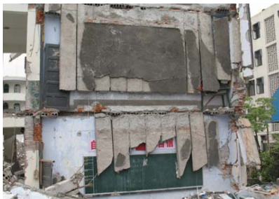
Figure 5. Collapsed floor planks
