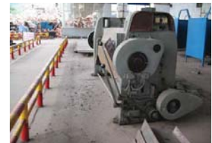
Figure 18. Sliding of un-anchored equipment
