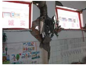
Figure 9. Captive column failure
