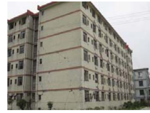
Figure 11. Cracked URM wall
