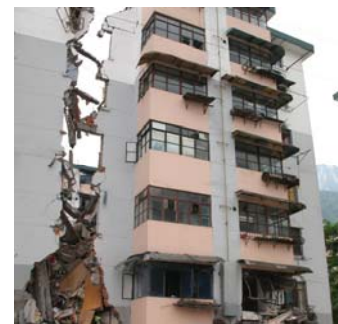
Figure 25. Vertical split and displaced apartment complex
