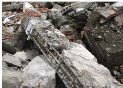
Figure 6. Collapse URM wall and concrete beam
