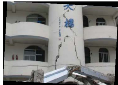
Figure 7. Shear cracks in masonry walls
