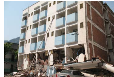
Figure 14. Soft story collapse
