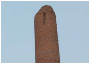
Figure 15. Damaged URM stack
