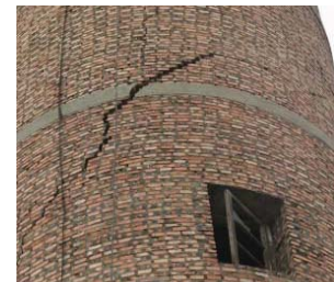
Figure 29. Shear crack in URM water tower
