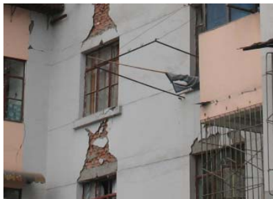
Figure 24. Cracked URM walls
