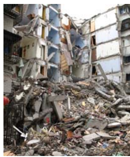
Figure 20. Collapsed corner of the building
