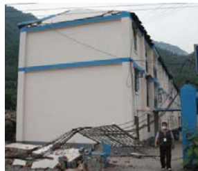
Figure 21. Damaged roof of the building
