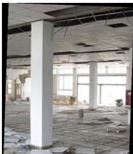
Figure 19. Damaged suspended ceiling
