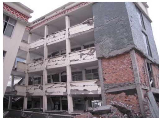
Fig6. the complex building of the Yingxiu secondary school (Local 1)
