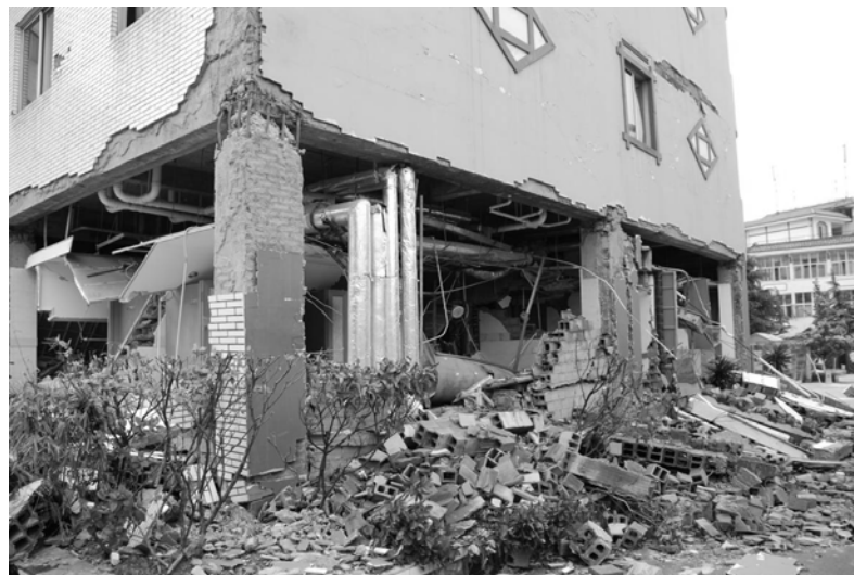
Figure 4: View of a building in Dujiangyan founded on river deposits with serious structural damages on the ground floor props. (type of building D, damage degree 4).
