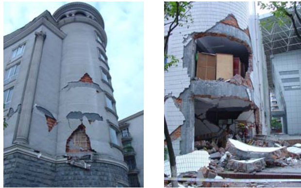
Fig. 16 Failure of walls at the corner of buildings (7/8)
