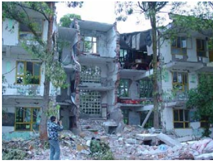
Fig. 9 Collapsed stair shaft of masonry school building in Mianzhu County (7/8~9)
