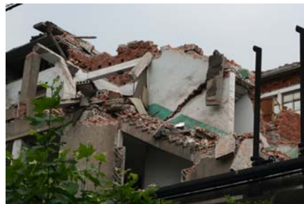
Fig. 12 The closely view of collapsed stair shaft (7/8)
