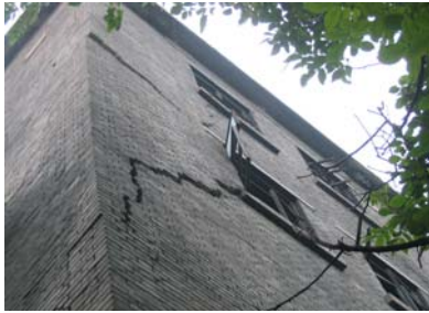
Fig. 15 Rotation at upper corner of a masonry building
