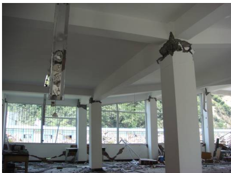
Fig. 5 Plastic hinges of the frame columns of Yingxiu School (7/11)
