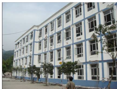
Fig. 8 Damaged school building of brick structure in Bailu (7/8)
