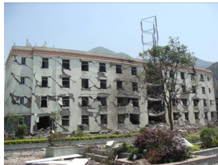
Fig. 2 Damaged office building in Yingxiu Town (7/11)
