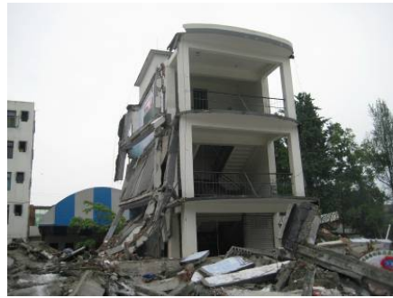
Fig. 10 Remained RC stair shaft of masonry school building in Dujiangyan County (7/8~9)
