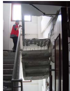
Fig. 14 Stair segment falling
