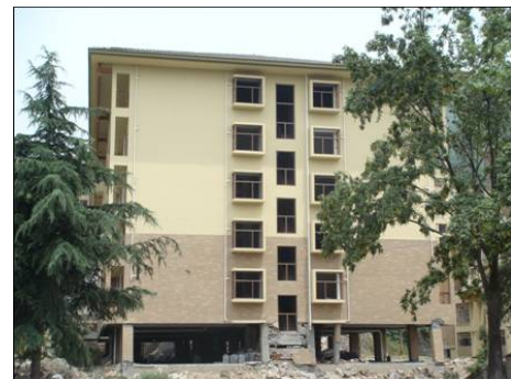
Fig. 6 Plastic hinges at top of columns of a residential building (7/9)
