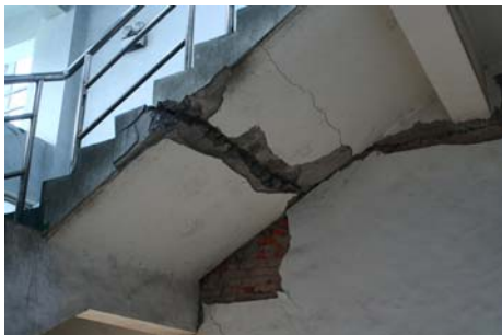
Fig. 13 Fractured stair beam at its lower 1/3 position (7/8~9)
