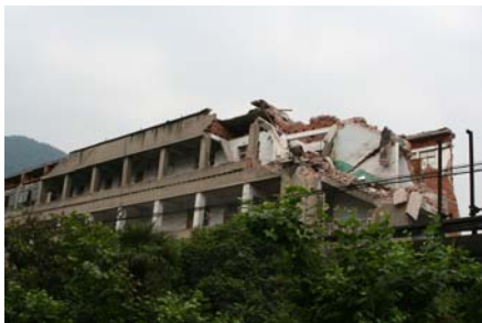
Fig. 11 Collapse of the stair shaft in the end of building plan (7/8)
