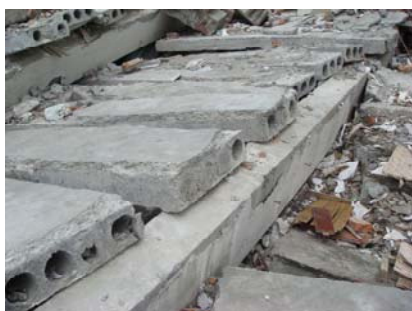
Fig. 7 Fallen RC beam and precast floor slabs in Pingwu (7/9)
