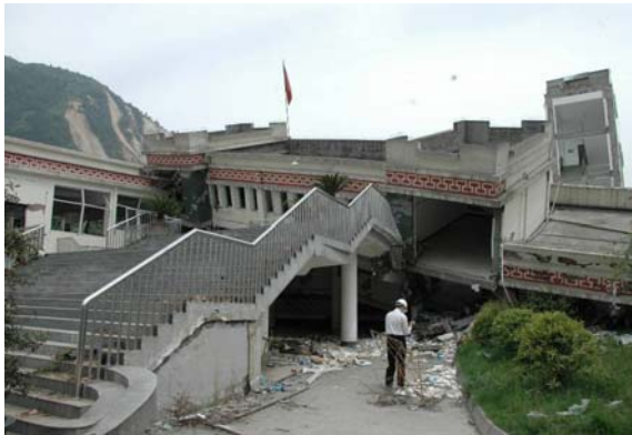
Figure 14 Total collapse of school building.
