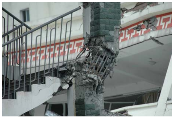
Figure 23 Column failure due to insufficient transverse reinforcement.
