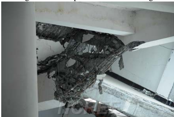
Figure 20 Column failure due to insufficient transverse reinforcement.
