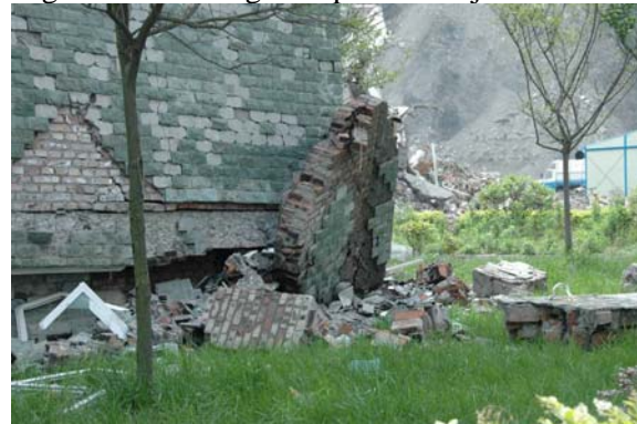
Figure 21 Soft story collapse.
