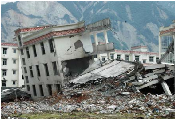
Figure 18 Collapse of school buildings.
