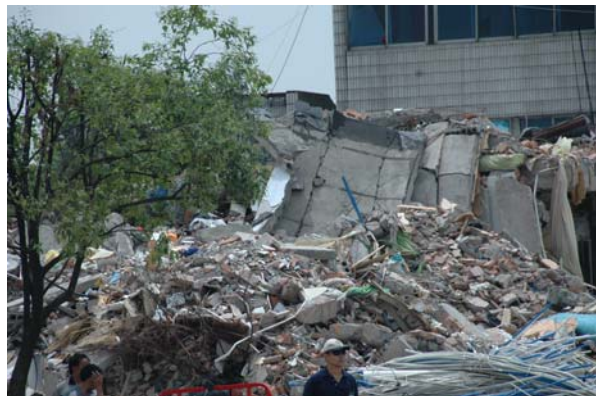
Figure 25 Building collapse of the 3 rd People's Hospital at Hanwang township, Mianzhu County.
