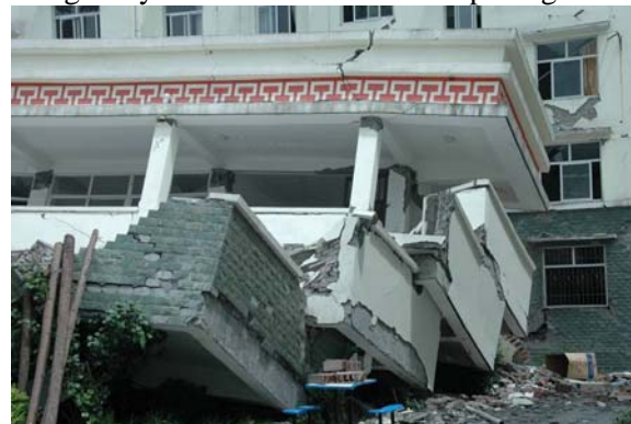
Figure 17 Pancake type of failure due to weak columns.
