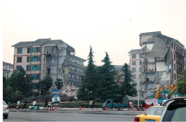
Figure 9 Partial collapse of commercial-residential buildings at Dujiangyan.
