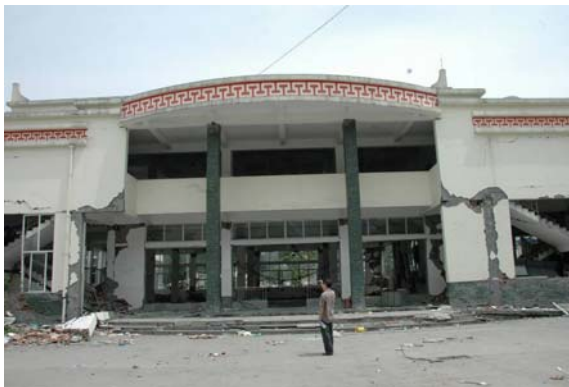
Figure 16 Severe damage of school building.
