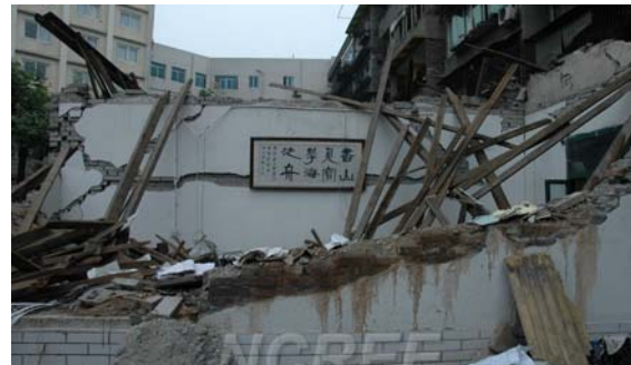
Figure 3 Collapse of elementary school building at Dujiangyan.
