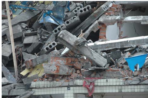
Figure 1 Photographical close-up view of the collapsed Employee Dormitory of the 3 rd People's Hospital at Hanwang township, Mianzhu County after earthquake.
