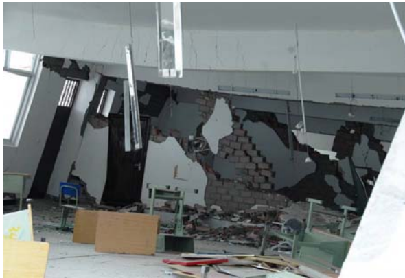
Figure 22 RC beam and nonstructural partition wall failure in the classroom.
