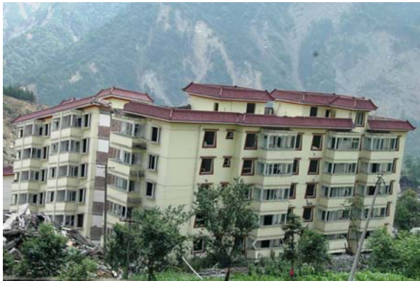
Figure 10 Soft story collapse of residential buildings at Yingxiu.
