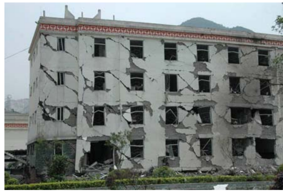
Figure 15 Severe diagonal shear cracks on the gravity wall between window openings.
