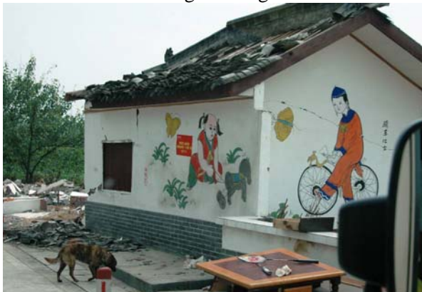
Figure 12 The black clay roof damage and wall cracking of a traditional house at Mianzhu.
