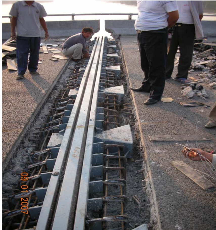
Fig. 9 (Shandong China Installation)
