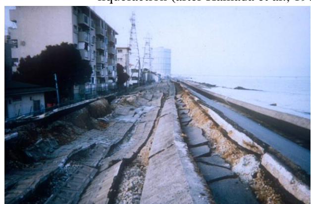
Figure 20 Damage of Yodo River dike during 1995 Kobe earthquake (Fudo Construction)
