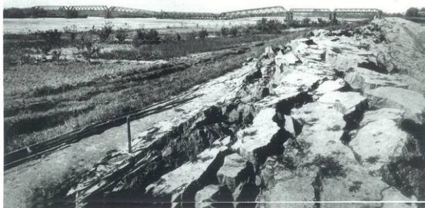
Figure 5 Damaged river dike (1891 Nobi earthquake)
