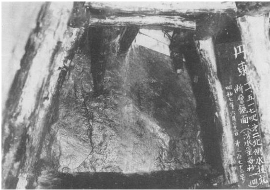
Figure 11 Fault plane that appeared in ongoing Tanna Tunnel project (Atami Construction Office, 1933)
