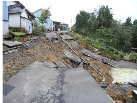
Figure 22 Collapse of fill on former valley topography (2004 Niigata Chuetsu earthquake)
