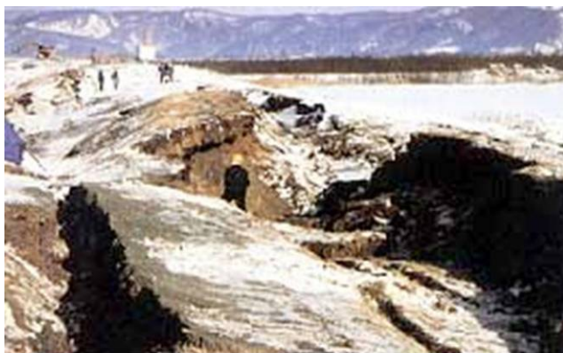
Figure 19 Damage of Tokachi River dike during 1993 Kushiro-Oki earthquake (Ministry of Construction)
