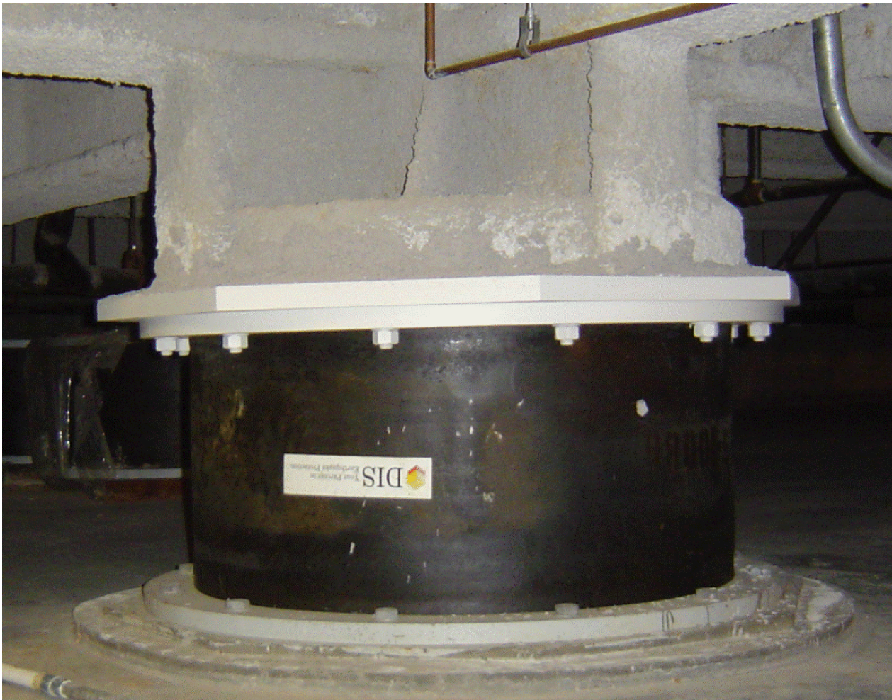
Figure 5 An installed NRB
