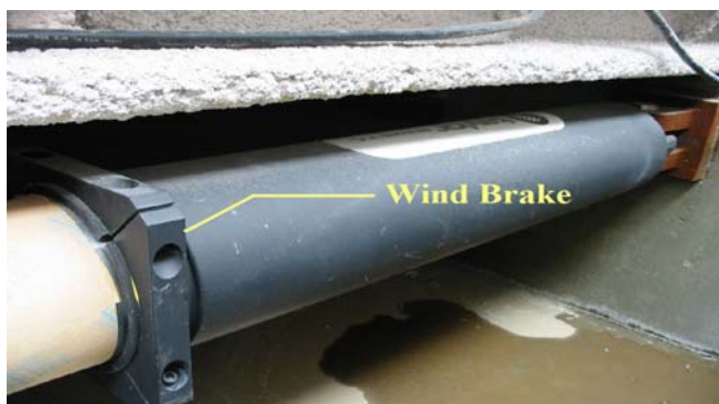
Figure 10 Installed 320kip VFD with wind brakes
