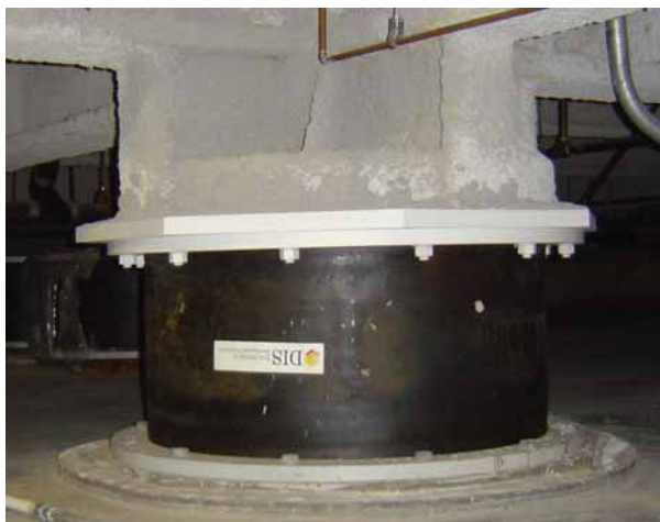
Figure 4 An installed NRB
