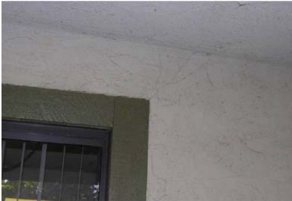
Figure 3. A typical damage observation: minor cracking in the stucco finish.
