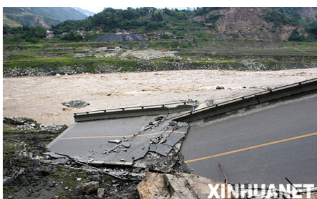
Fig. 2 The collapsed White Flower Bridge
