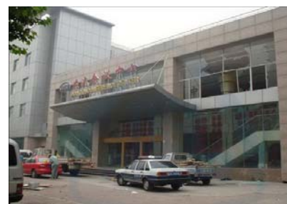
Fig. 3 The frame-structure building with little damage
