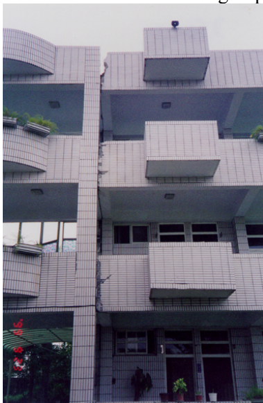
Figure 1 Ponding damage due to insufficient seismic gap
