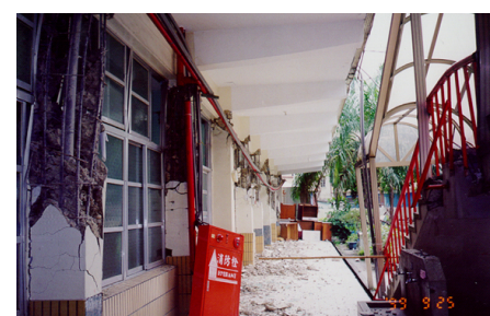
Figure 3 Short column damage
