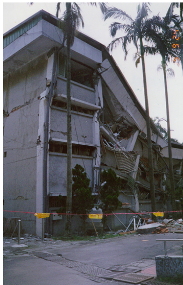
Figure 2 Earthquake damage due to vertical building expansion
