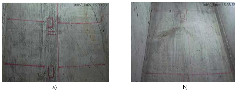
Figure 6 Internal damage in the West web for 0.93% drift: a) PO2-N5 and b) PO2-N6
