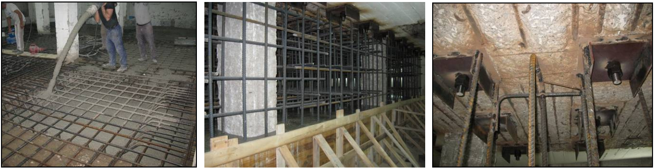
Figure 6 Grid foundation plate and casting of the concrete (left); spatial grid of the reaction mass (centre); details of the welding (right)
