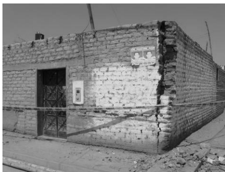
Vertical crack at corner of front wall
