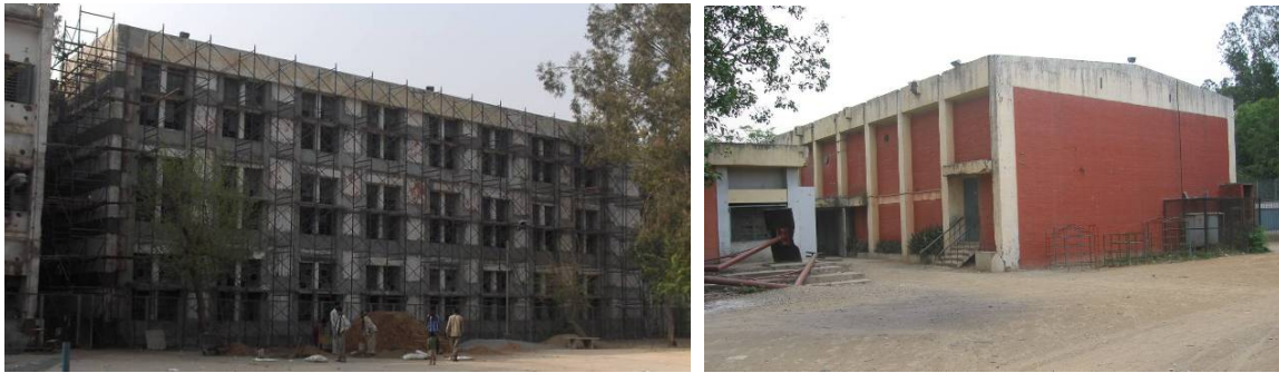
Figure 2. Ludlow Castle School classroom block undergoing retrofit (left) and multipurpose room (right)
