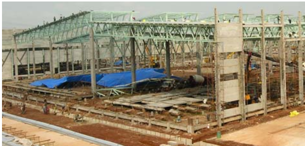
c. PC columns, beams and HCS with 70 mm topping at Main Factory Building
