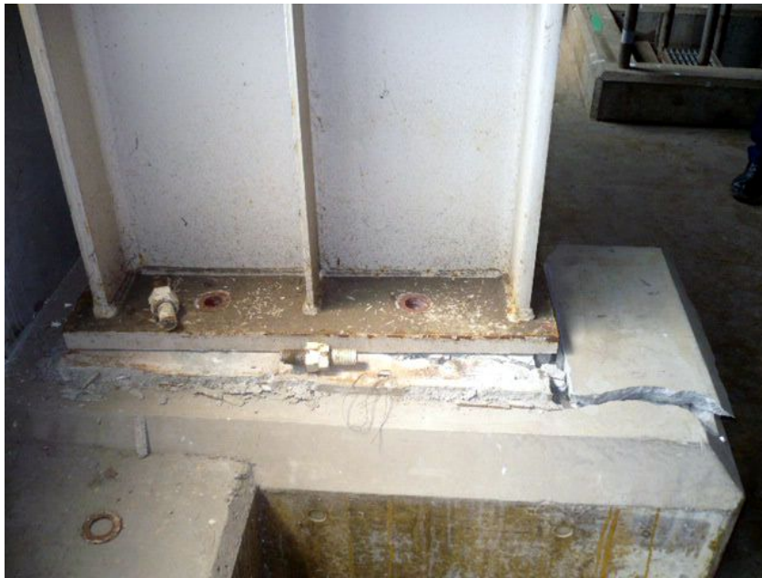
Figure 7 Damage of bolts in a C class building by courtesy of TEPCO
