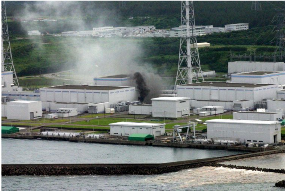
Figure 1 Fire of a transformer by courtesy of 9 th Regional Headquarters of Japan Coast Guard
