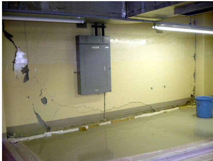
Figure 4 Cracks on the underground RC wall of a C class building produced by earth pressure by courtesy of TEPCO
