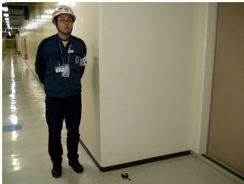
Figure 8 RC wall 1.5m thick of an A class Reactor building The thickness was decided by the earthquake force 0.48G, 3 times of C class building. by courtesy of TEPCO
