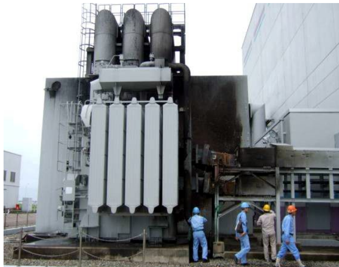
Figure 2 After the fire of the transformer You can see the fire convention wall behind the transformer, change to dark color by smoking. by courtesy of Tokyo Electric Power Co. (TEPCO)
