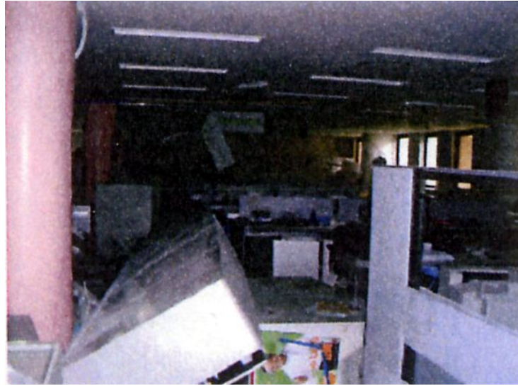
Figure 5 Falling down of various things inside of a C class building by courtesy of TEPCO
