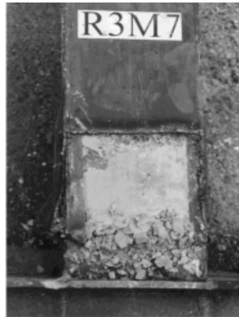
Fig.5 Typical concrete failure Appearances of Filled-in Concrete
