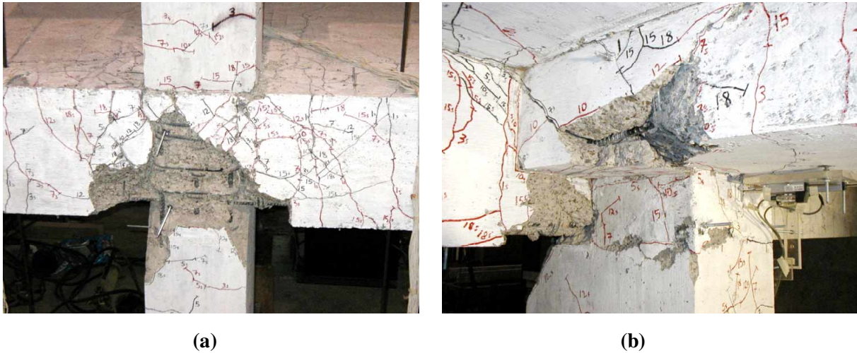
Figure 7: Cracking Pattern at the (a) Exterior and (b) Interior Faces of Specimen 3
