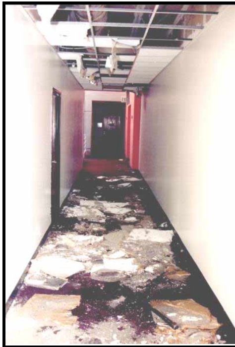
Figure 5 Drop-down ceiling contact resulting in fire sprinkler system damage Northridge earthquake 1994
