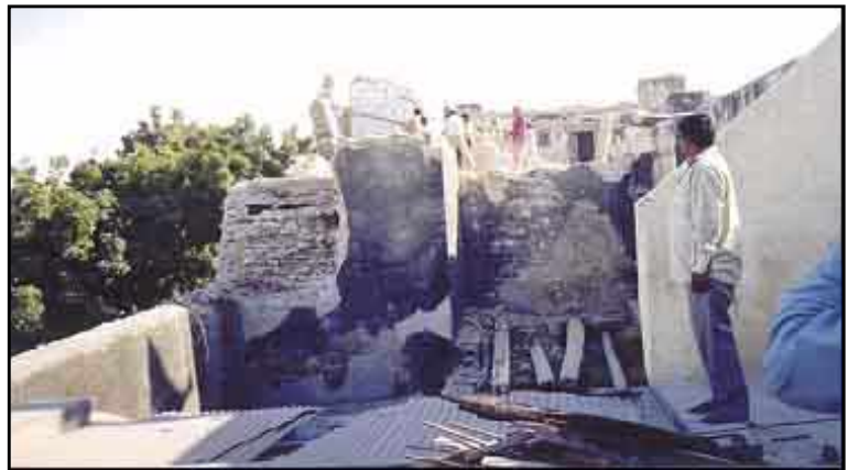
Fig. 7 Severely damage Beyt Dwarka temple.
