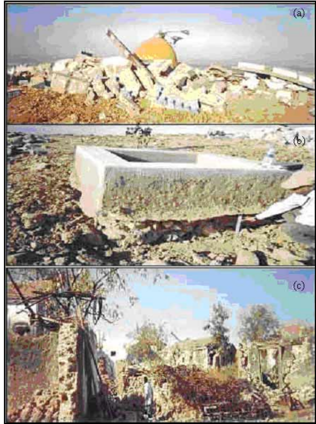
Fig. 4a. Collapsed temple situated on the top of Ram Dev Pir hill, b. Uprooting of water tank situated on the Ram Dev Pir hill and c. Damaged Kutri village situated on an elevated ground
