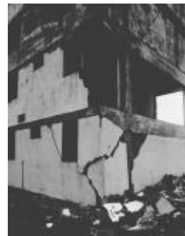
Figure 12: Damaged south-eastern corner of the building after the 1997 earthquake
