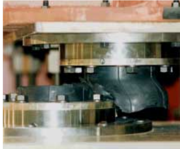
Figure 17 Sheared off flat rubber bearing
