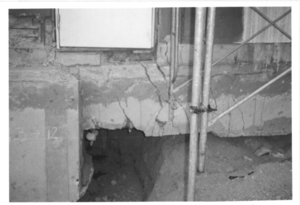
Fig.5 Cracks of strap beam
