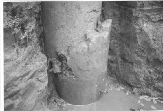
Fig.15 Damage of precast prestressed concrete piles, CASE C (shear failure, building B)
