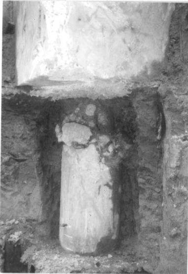
Fig.14 Damage of precast prestressed concrete piles, CASE C (Compressive failure, building A)
