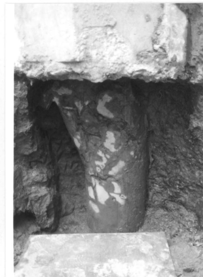
Fig.17 Damage of precast prestressed concrete piles, CASE C (Soil moved and pile head remained)
