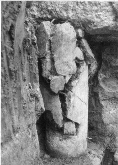
Fig.16 Damage of precast prestressed concrete piles, CASE C (shear failure + compressive failure, building C)
