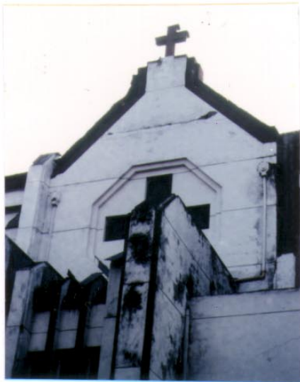
Photo 3. Ornaments fell off the Balbanera Church.
