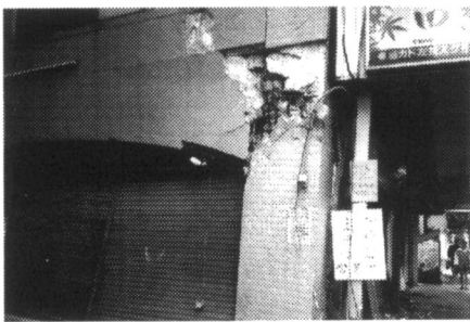
Photo 5. A single span RC building with heavily damaged exterior joint at 2nd floor
