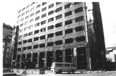
Photo 4. An 11-story SRC City Office building with damaged secondary walls and severe damage of joints
